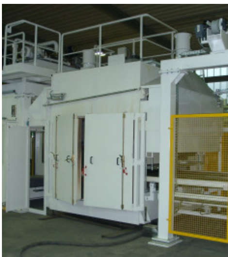
Heating oven for vehicle insulation mats
